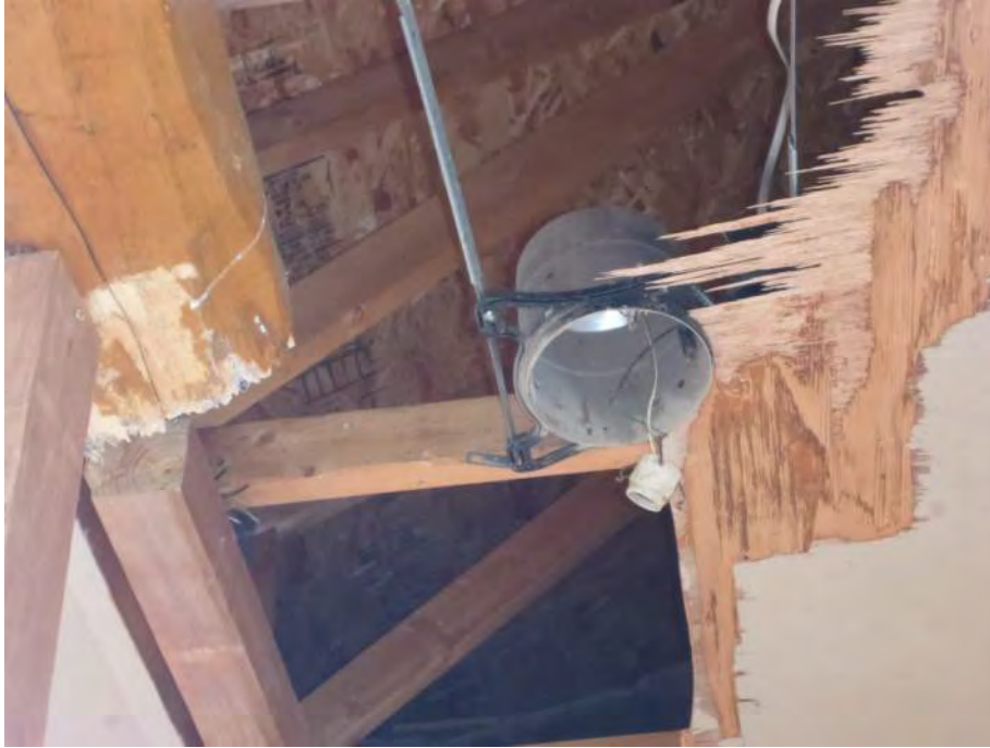
Figure 11. Damaged can light and missing fixture adjacent to impact damage on west log beam
