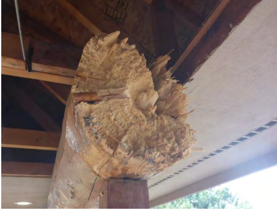
Figure 7. Fractured north end of remaining portion of west log beam
