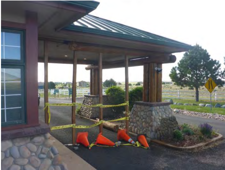
Figure 3. Overview of impact damage to north end of west log beam with temporary shoring in place (looking southeast)
