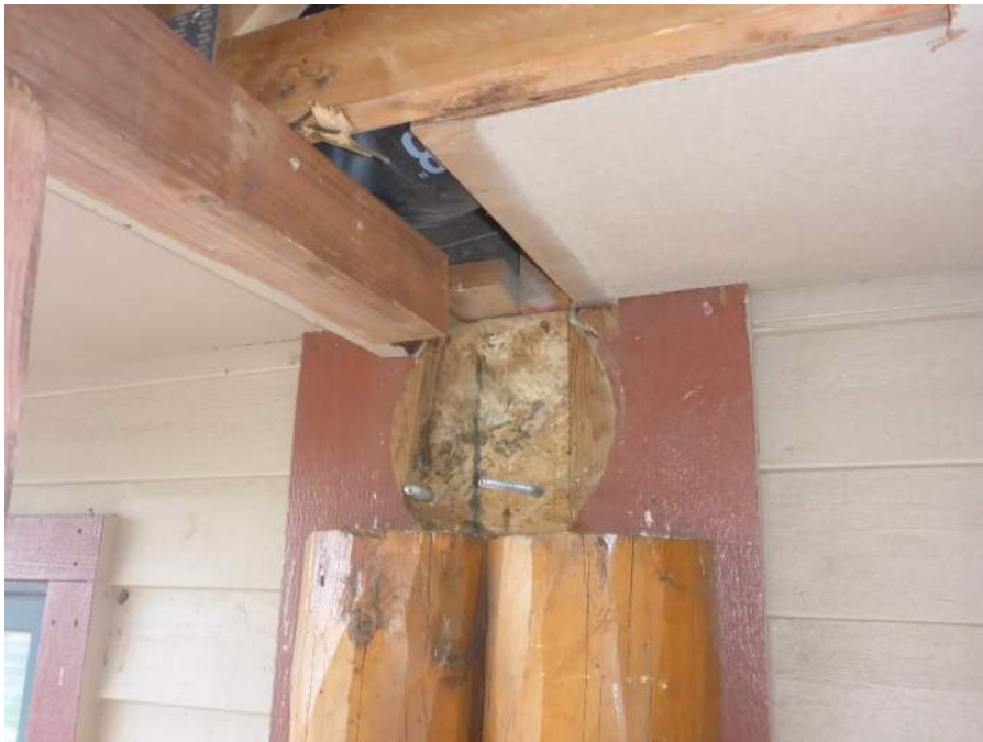
Figure 6. Bearing connection at north end of west log beam
