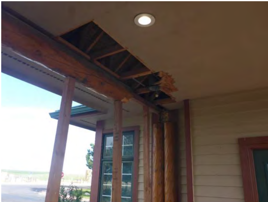
Figure 4. Overview of impact damage to north end of west log beam and adjacent soffit sheathing (from southeast)
