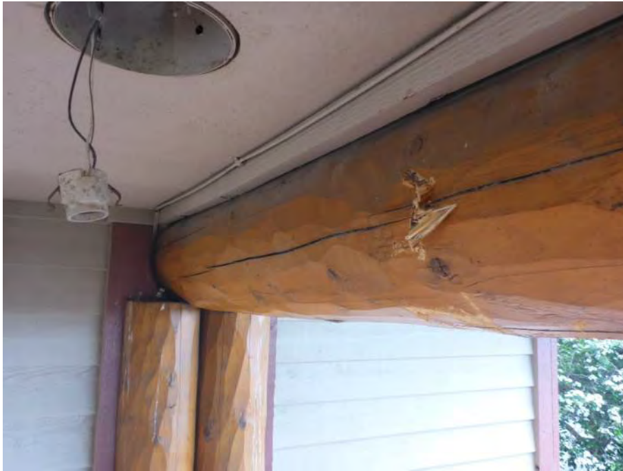
Figure 9. Overview of impact damage to east log beam, approximately 4'-4" from north end
