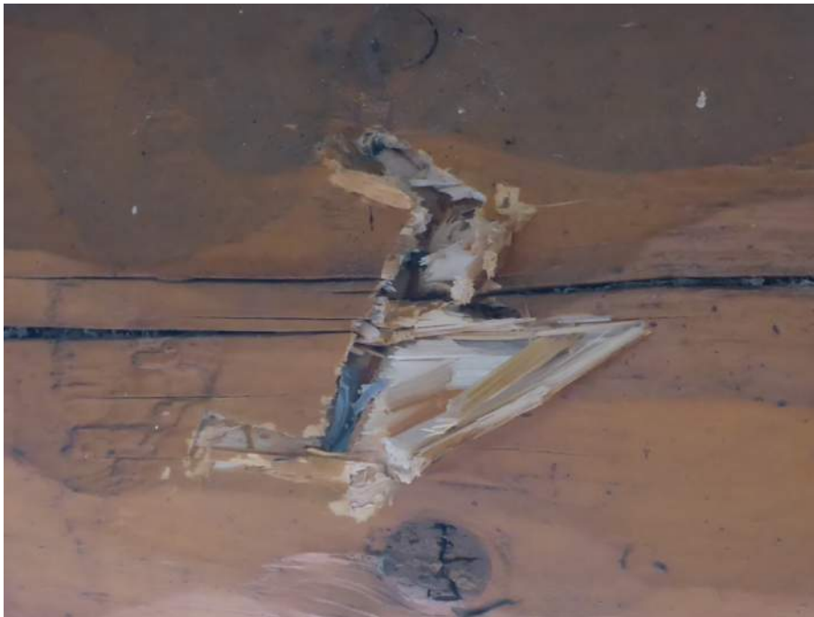
Figure 10. Close-up of impact damage to east log beam
