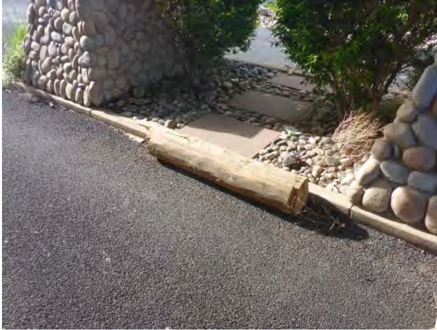
Figure 5. Fallen portion from north end of west log beam
