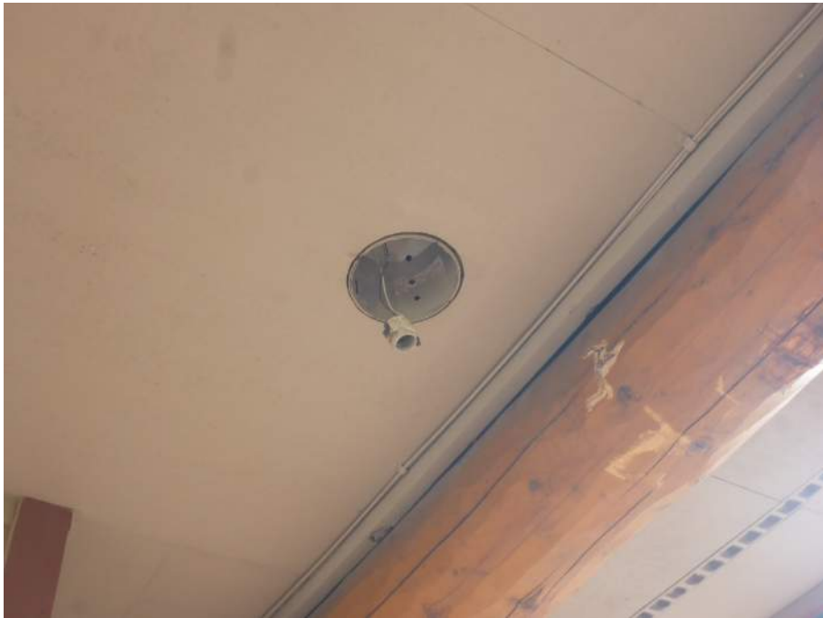
Figure 12. Missing light fixture adjacent to impact damage on east log beam
